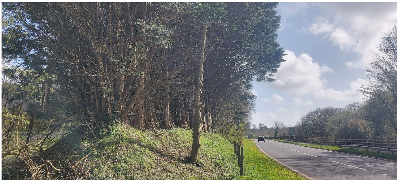
Photo of man made embankment and lean of trees
